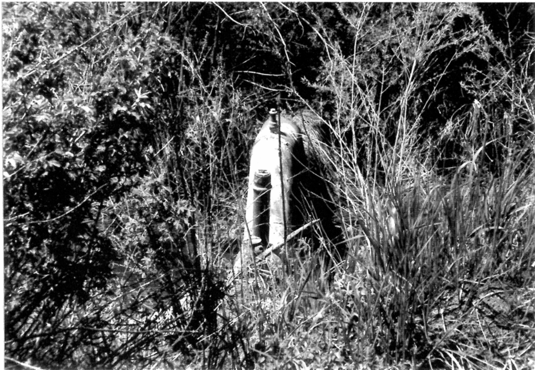
Pipe Further Along for Gravity Flow
